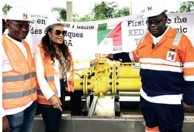
Commissioning of the gas pipeline supplying natural gas to a tile factory
